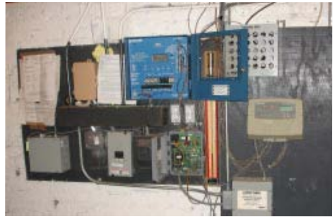
116 Heat-Timer Platinum weather actuated controls were installed in Beach Lane Management properties.
