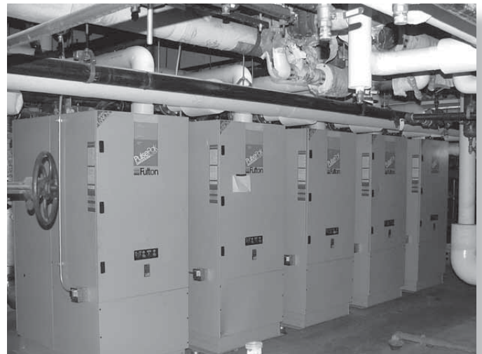
A Heat-Timer Multi-Mod with an extension module provides modulating and lead lag control for five pulse boilers.
